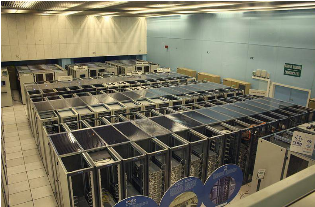
The CERN datacenter with World Wide Web and Mail servers
